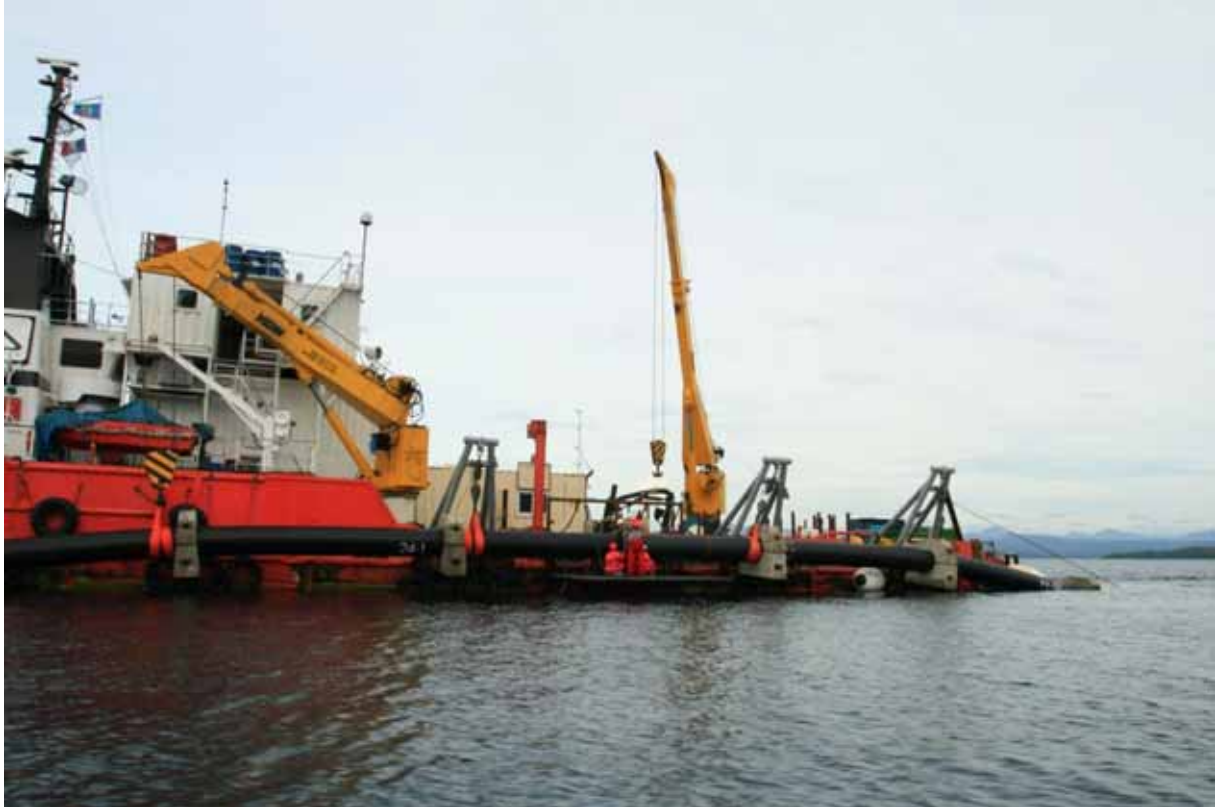
Figure 8: vue plus large du raccordement
